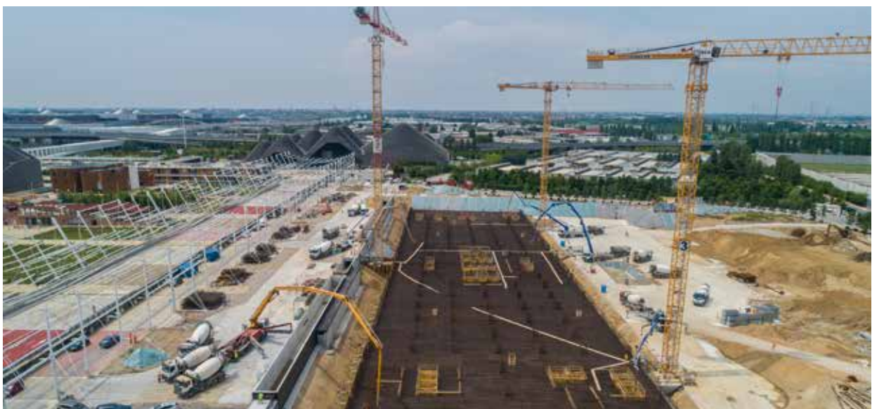
Work on the construction of the new headquarters of the Galeazzi Orthopaedic Institute in the former Expo 2015 site, Milan.
